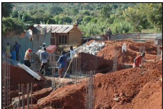
The foundation is dug and footings for the new building are put into place.
